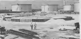
IN VARIOUS stages of construction in the tank farm the three huge gasoline storage tanks. Largest has a capacity of 80,000 barrels. All are floating-roof tanks because of special features incorporated in their design, the tanks can use a slightly thinner steel plating. New roof seals are more efficient in minimizing the evaporation of gasoline products.
